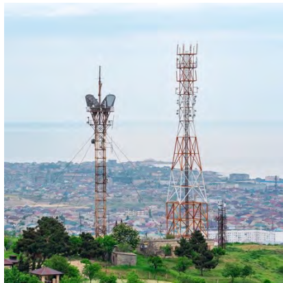
Telecom Base Station
